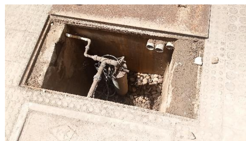
FIGURE 4: RAIN WATER HARVESTING
